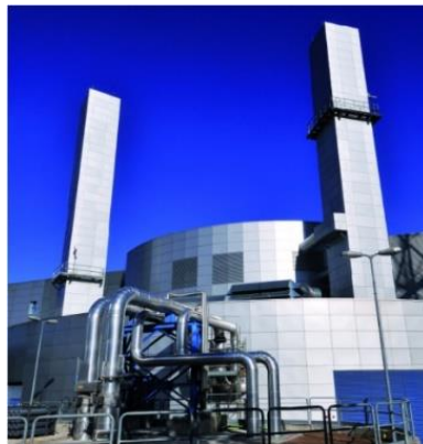
Figure 5. 10 MW district heating facility in Milan, Italy (Modern Power Systems, 2018).
